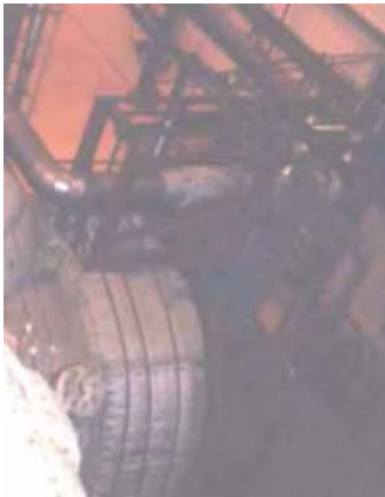
Figure 4: Gas detectors above a silo combustor.
