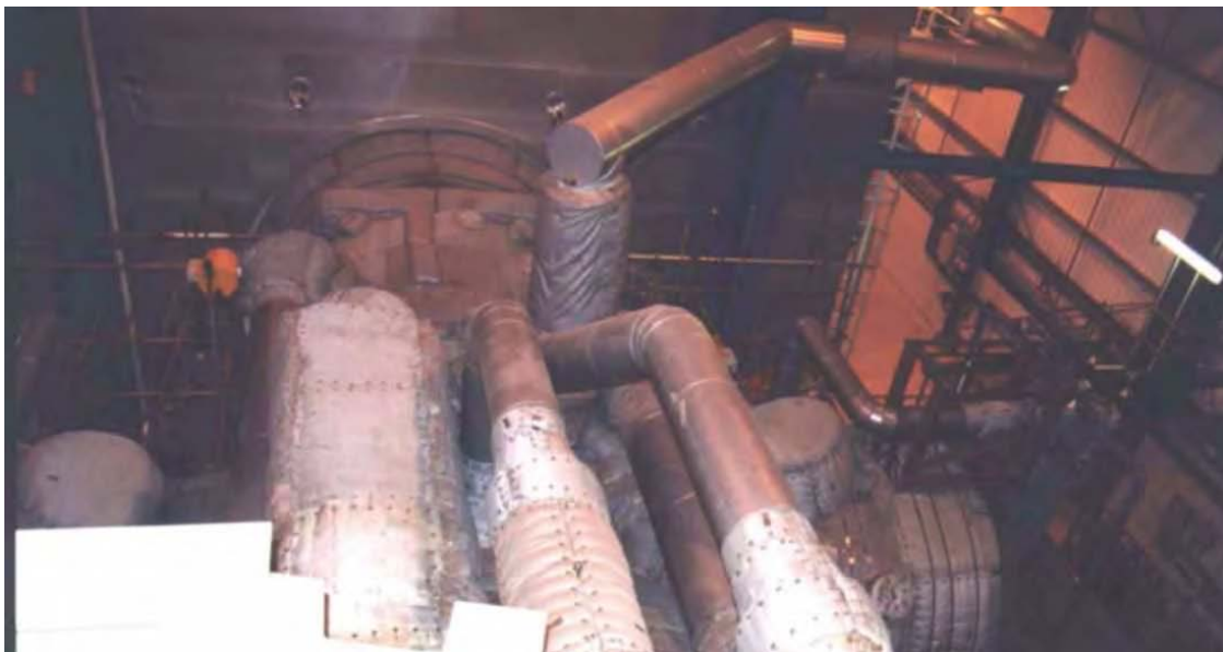
Figure 2: Pipework above a gas turbine.
