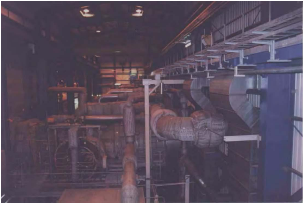
Figure 1: The gas turbine hall
