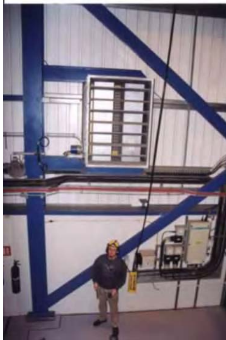
Figure 5: Inlet ducts with horizontal baffles, as found in the generator bays
