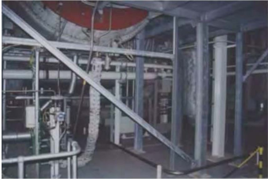
Figure 3: Pipework and structure beneath a gas turbine.
