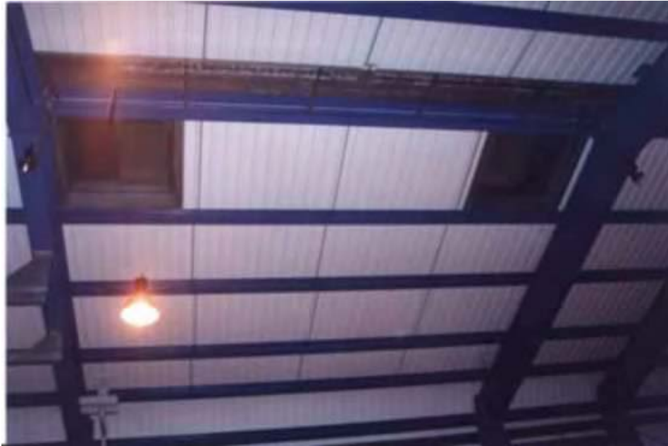
Figure 7: Roof extract ducts.
