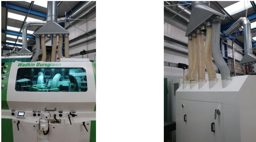
Figure 15 Dust extraction system (left: front view, right: rear view)
