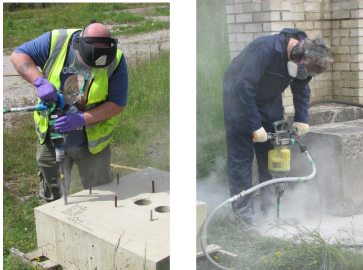
Figure 7. (a) Drilling vertically into concrete block, and (b) drilling into reinforced concrete pad
