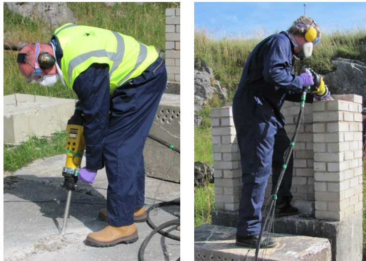
Figure 5. (a) Breaking the concrete pad (left) and (b) demolishing a brick wall
