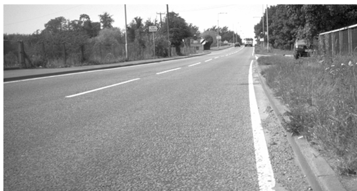
Plate 1: View of the road where the study was carried out, looking north showing debris in the gutter
