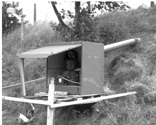
Plate 3: Overview of the monitoring installation
