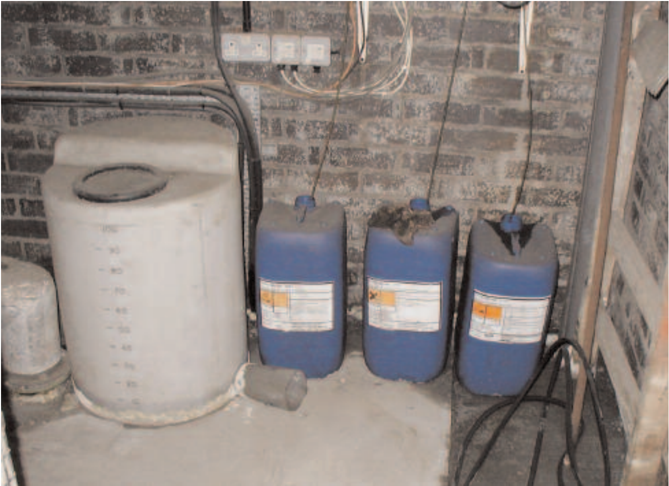
Figure 7 The two biocide and one anti-scale and corrosion chemical drums
