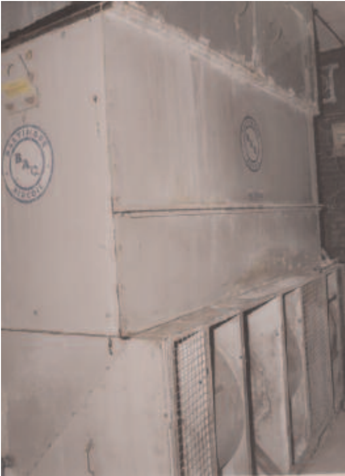
Figure 4 (Left) Cooling tower 1
