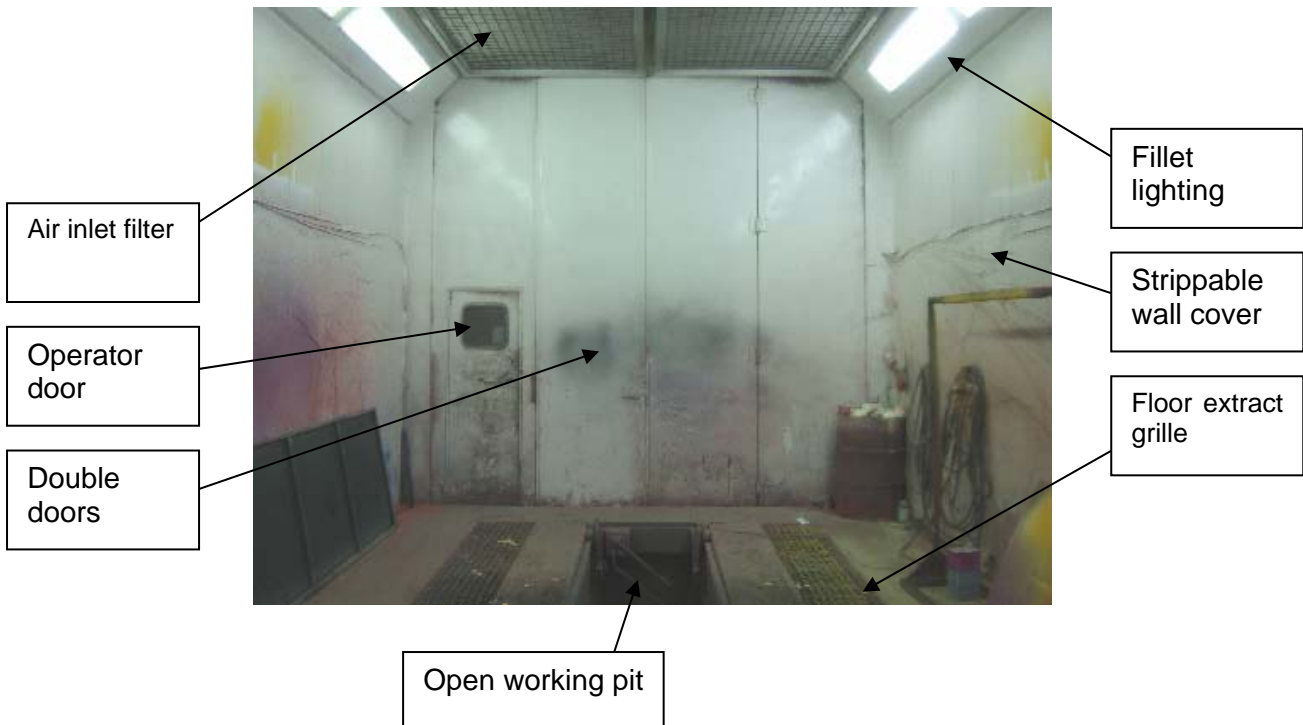
Figure 5. Photograph of a booth featuring double doors, personal operator door, open working pit, air inlet filters, floor air extraction filters and grille, strippable wall cover and fillet light panels. Normally the pit should be covered when not in use.
