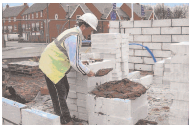
Figure 3 Raising the height of a mortar spot board reduces the risk of injury from repeated bending
