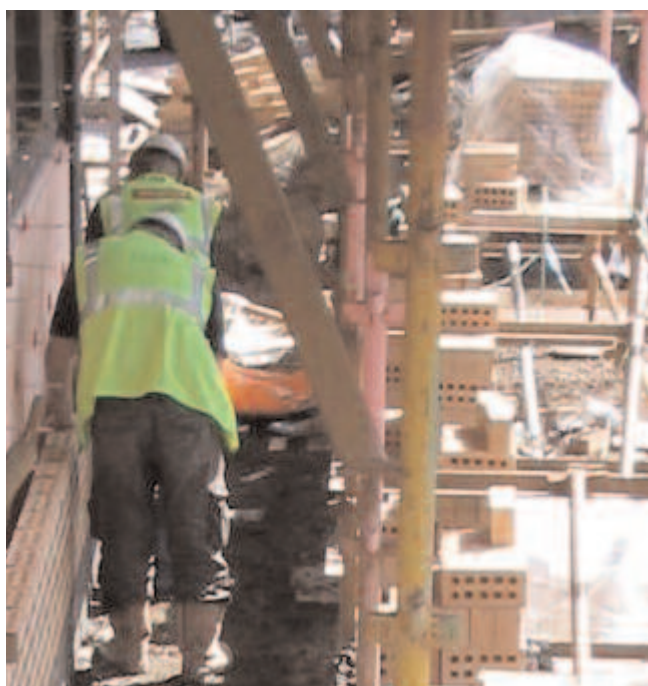
Figure 2 Stacks of brick are placed on the scaffold to raise their height and reduce the need to bend
