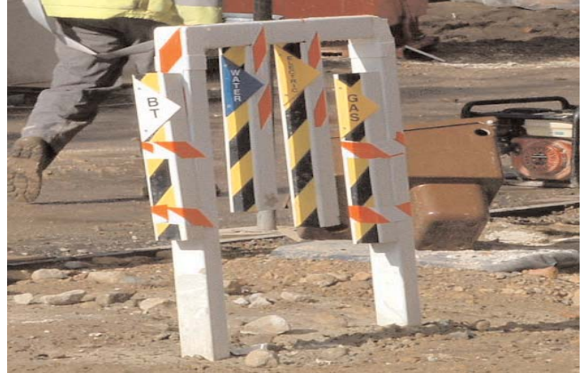
Figure 3 A site service marker
