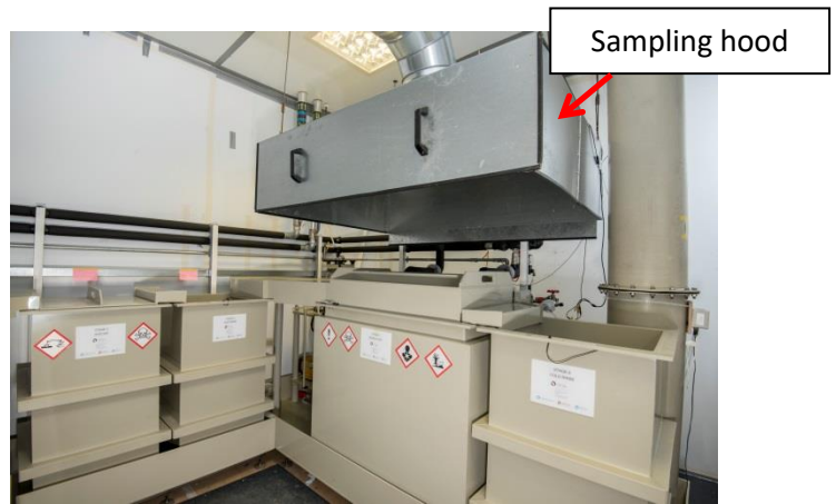
Photograph 2. Overview of plating line, view 2.
