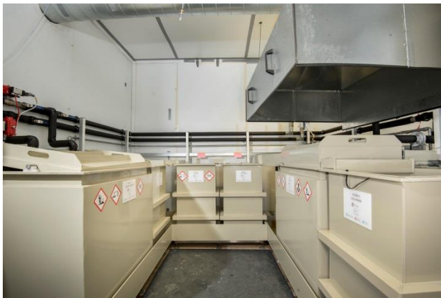
Photograph 1. Overview of plating line, view 1.
