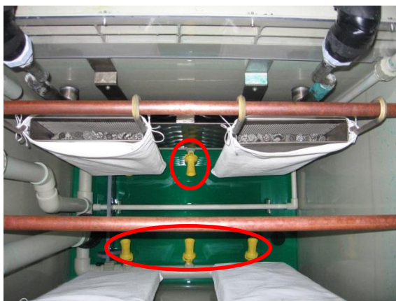
Photograph 4. Arrangement of eductors (circled). Note there are a total of six, three each side all angled upwards (two obscured by anode baskets).
