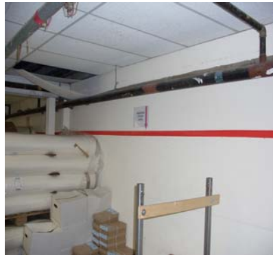
Photograph 10. The painted red line indicates that products should not be stored above it
