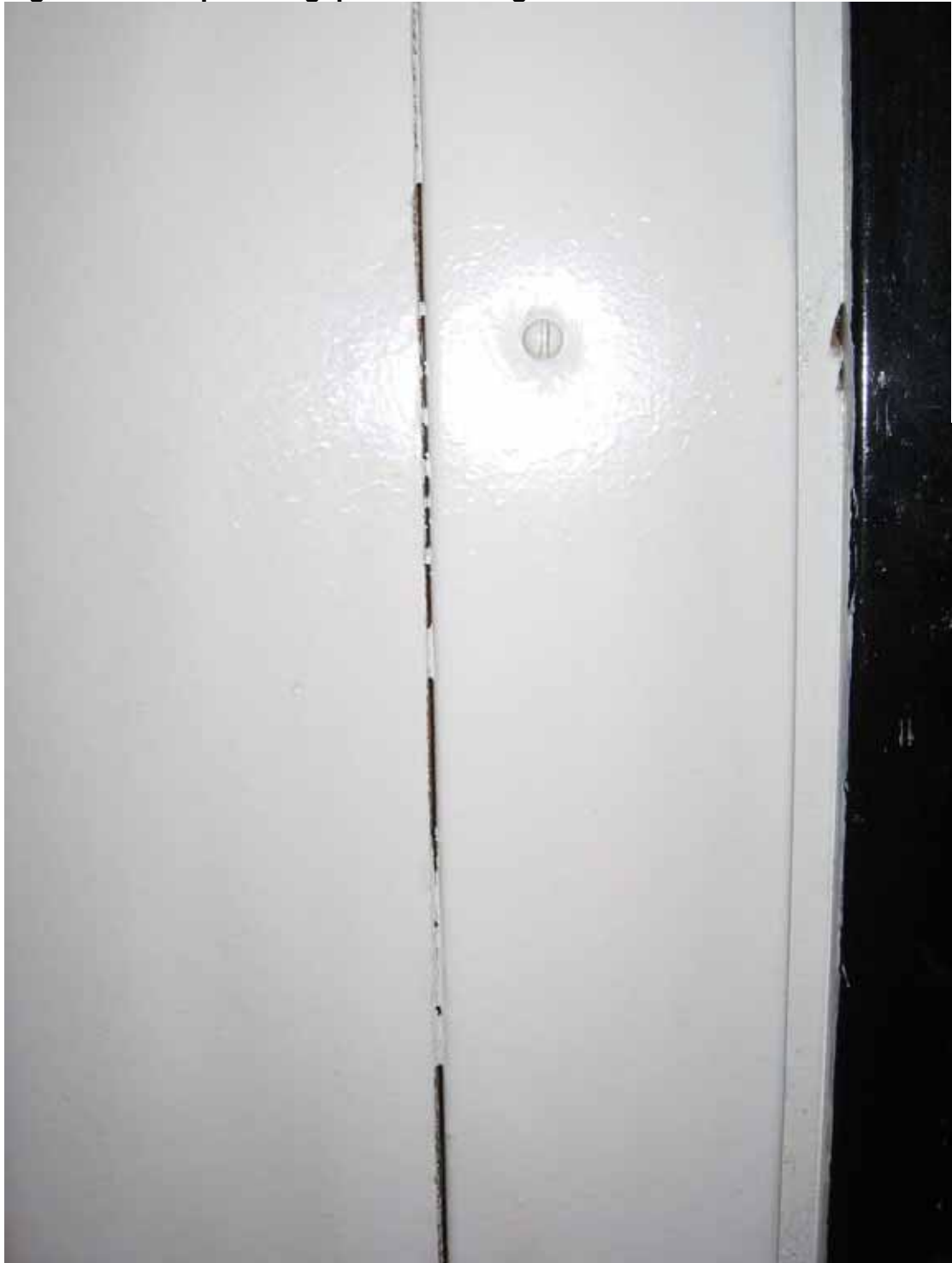
Figure 4: Example of a gap in the casing
