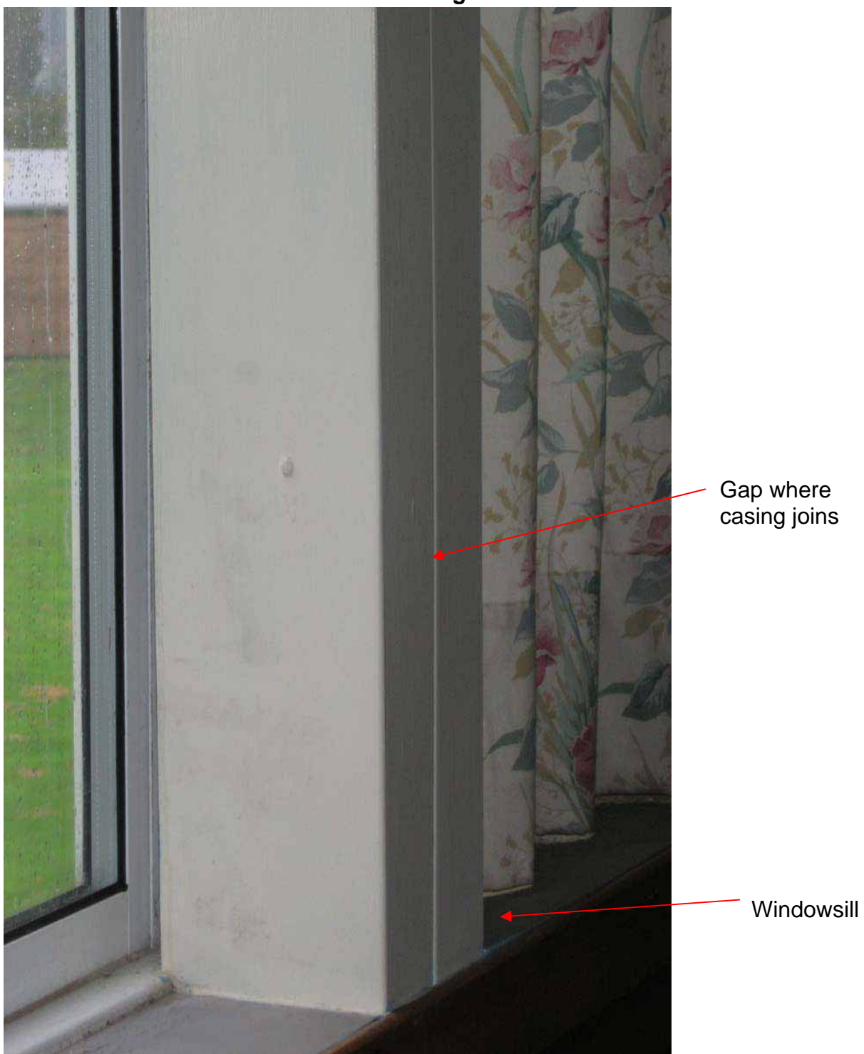
Figure 2: Metal clad column showing gap at front of column where the two halves of the cladding meet
