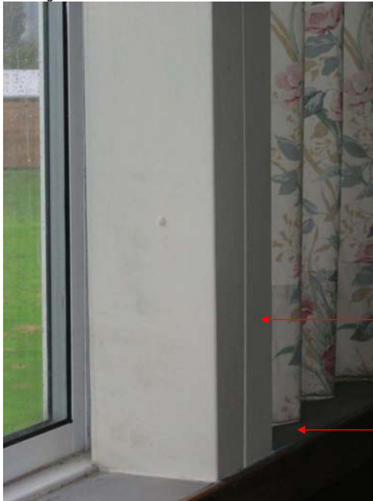
Figure 2: Metal clad column showing gap at front of column where the two halves of the cladding meet
