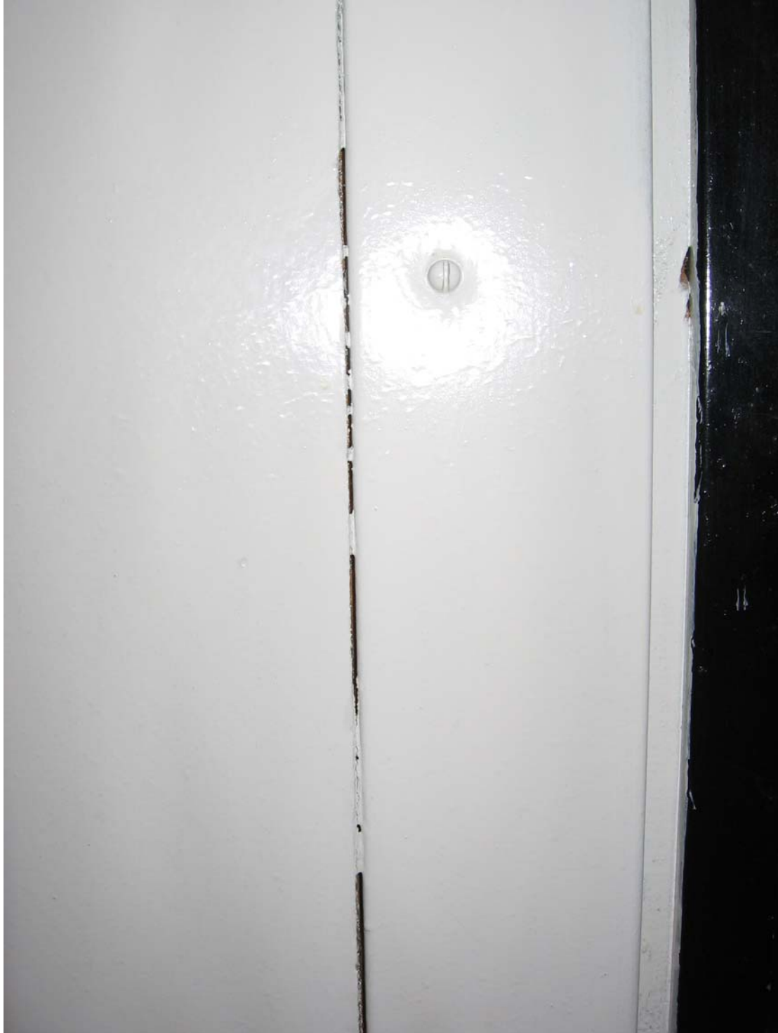
Figure 4: Example of a gap in the casing
