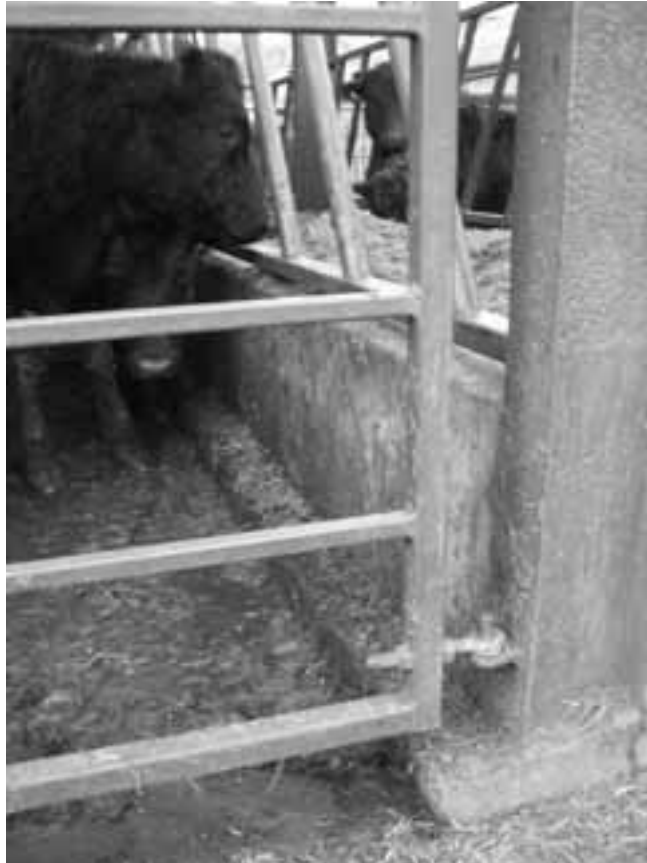
Kerbs to protect gates during slurry scraping
