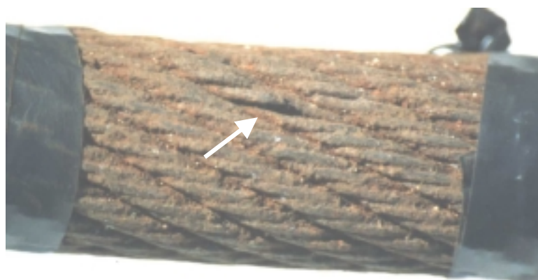
Figure 1 Typical external condition of the rope in the as received condition (length 1: 18.33m) (Note the wire break in the middle of the figure)
