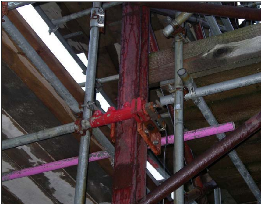
Figure 7 - Modified Instrumented Tie
