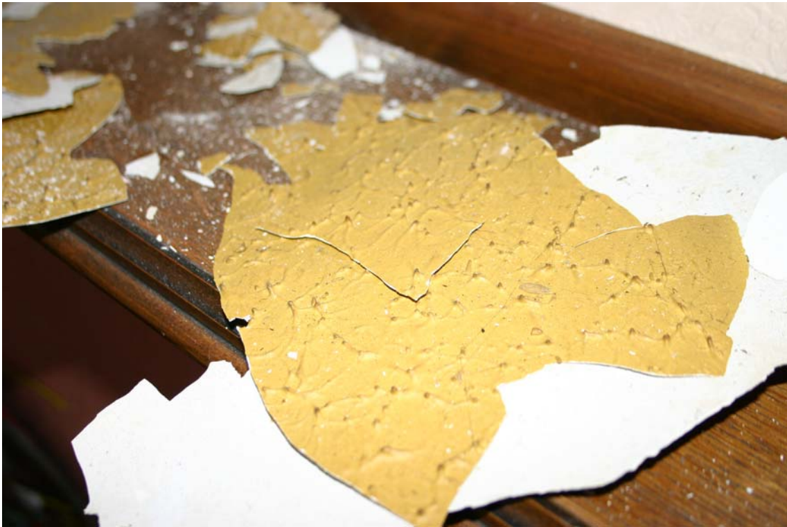
A2:2 Photograph of large pieces of the TDC. These had fallen from the ceiling during the dismantling of the false ceiling.
