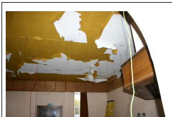
Figure 2: The ceiling in the area where the TDC was in very poor condition. The end of the bar area can be seen on the right and thin metal wires from which the false ceiling hung are visible.
