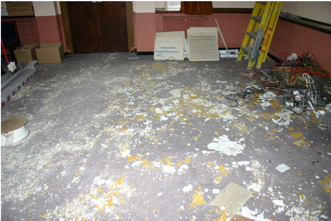
A2:3 Photograph showing high concentrations of contamination much of which was TDC from the ceiling.
