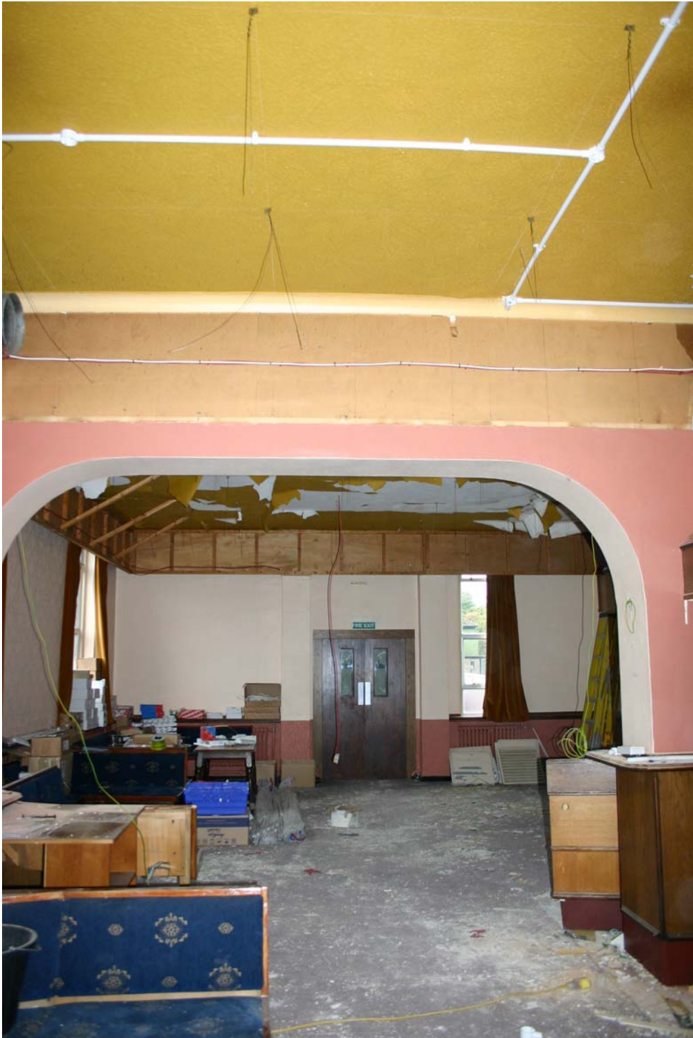
A2:1 View of bar area after removal of false ceiling. All the movable items were removed prior to stripping the ceiling. The blue inserts were removed from the seats and the carpet and curtains disposed of. An airlock was built in the doorway at the end of the room and the bar area sealed off using plastic sheet.
