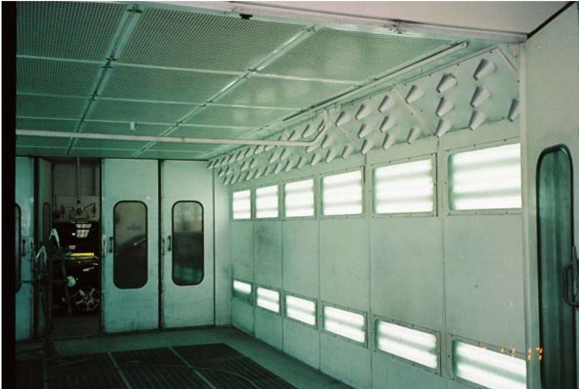
Figure 2: Company Six Spray Booth
