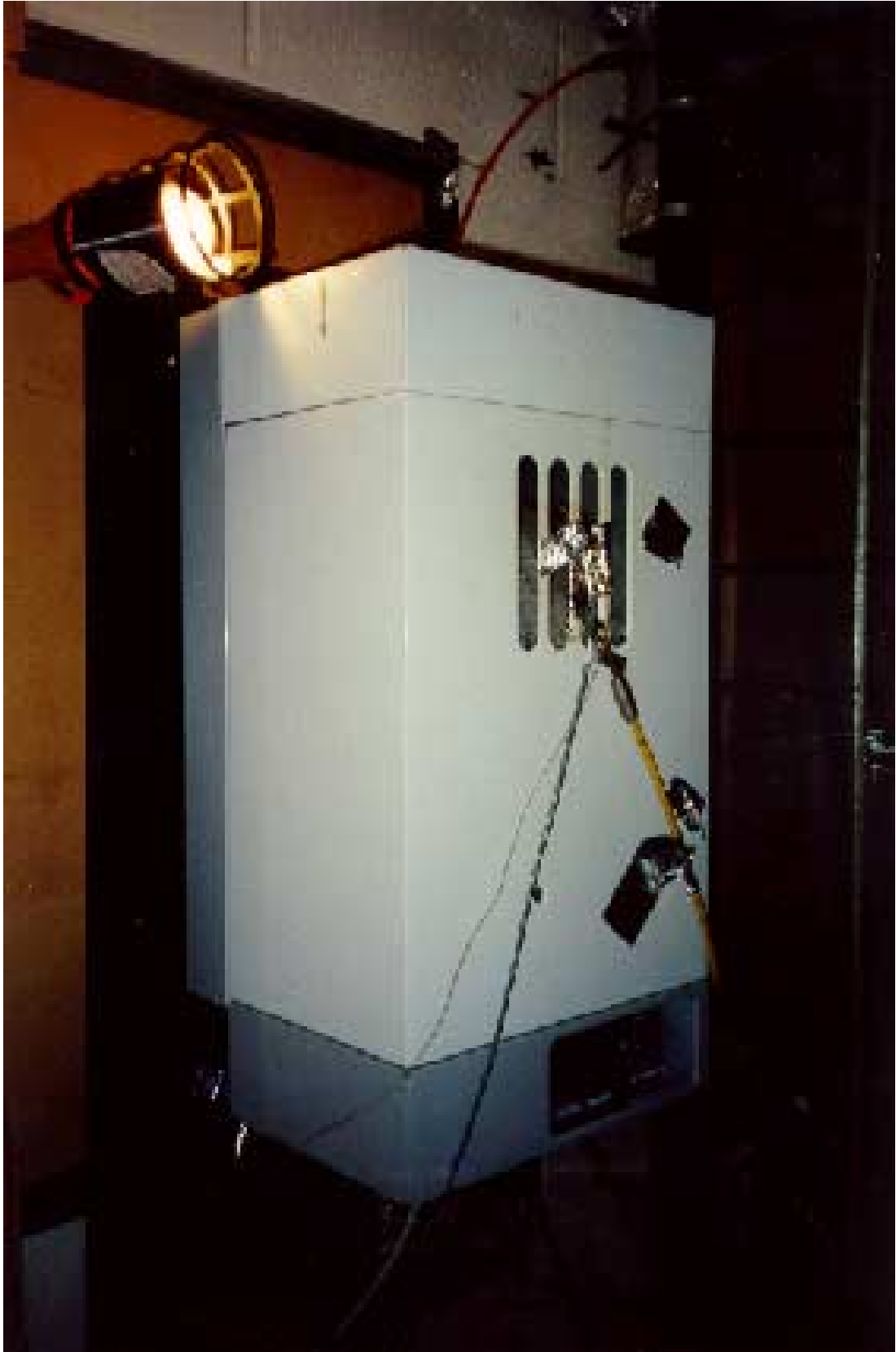
Figure 1: View of Boiler Inside Compartment Showing Sampling Positions at Draught Diverter
