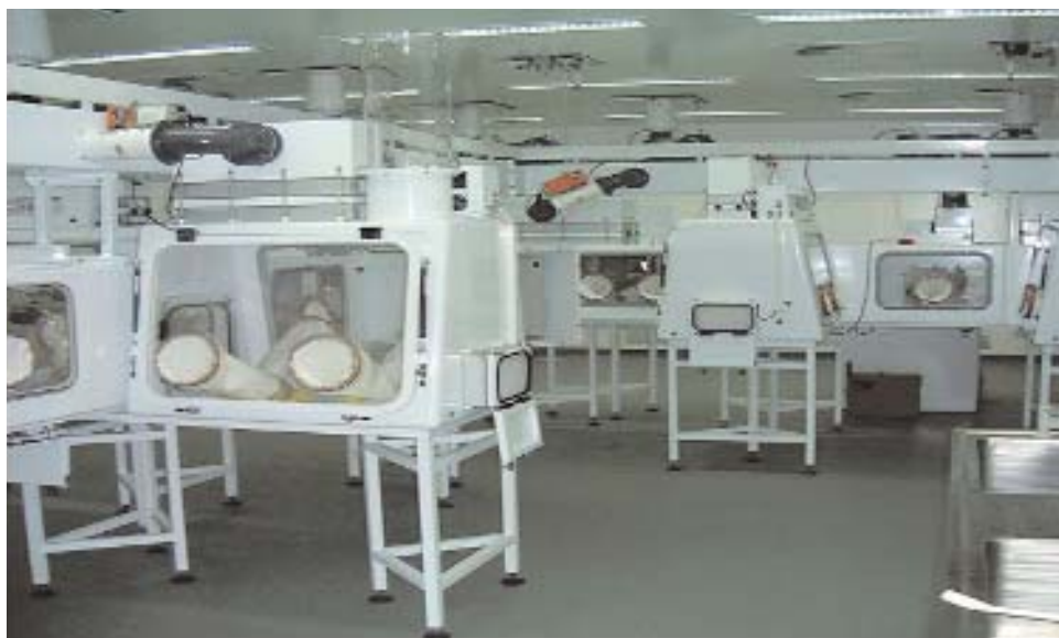
Figure 3: A cabinet line
