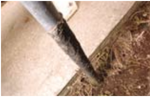
Metallic pipework protected as it enters the ground
