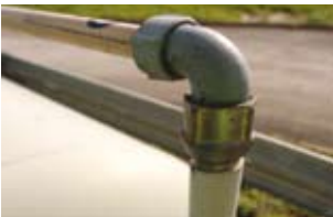
Pipework protected from below ground to emergency control
