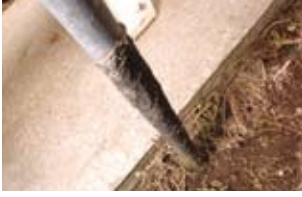
Metallic pipework protected as it enters the ground
