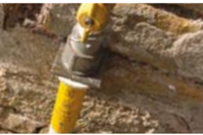
PE pipework protected from the last collar before entering the ground
