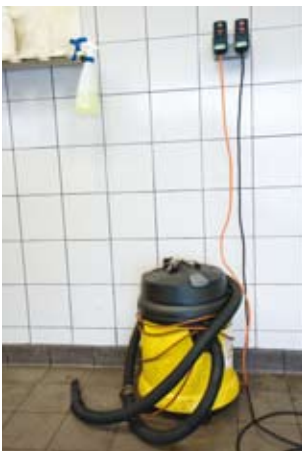
RCD protection provided for portable vacuum cleaner
