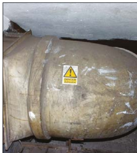
This section of AC ducting has already been labelled
