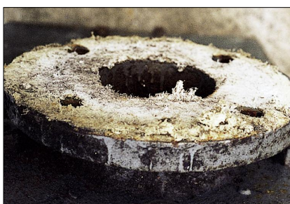
Gasket material left on a pipe flange
