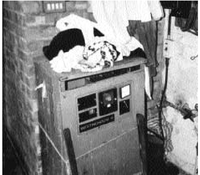
Electrical equipment housing held closed with string
