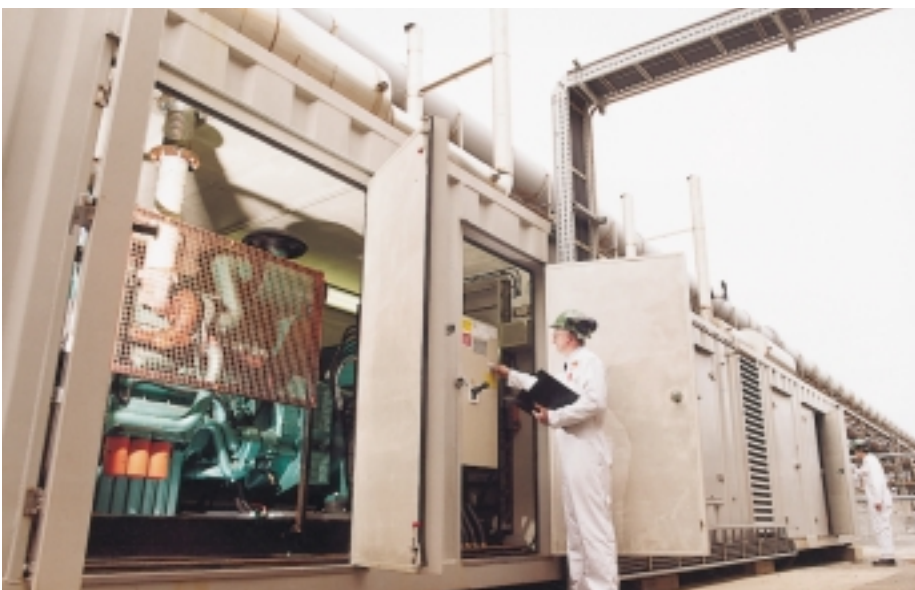
Two new 800kVA diesel alternators in weatherproof enclosures. Installed and engineered to provide back-up electricity supply to the fuel cycle area ventilation system fans.
