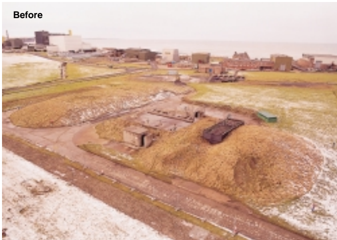
Redundant oil tank compound prior to excavation to remove the seven tanks that were installed when Dounreay was an airfield during World War II.
