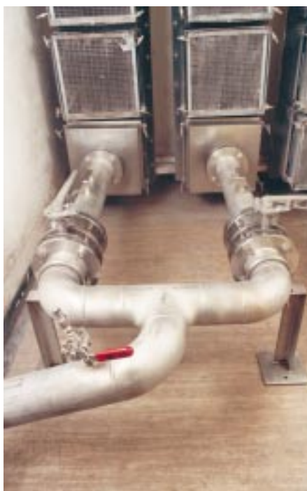
D9867 ventilation improvements
