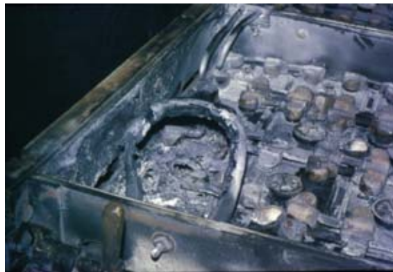
The aftermath of a fire in a lead acid battery following a short-circuit
