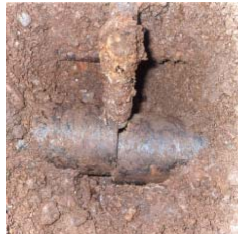
Figure 5 Picture of Fractured Main
