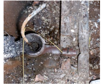
Figure 6 Electricity Duct with flexible tape inserted in air gap and electric cable rising inside to electric meter
