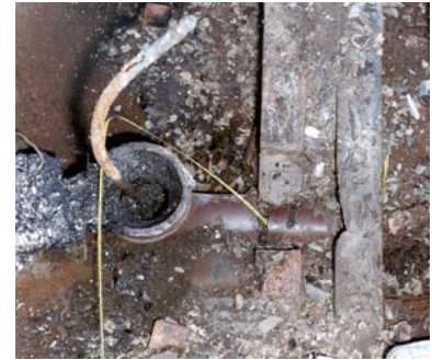
Figure 6 Electricity Duct with flexible tape inserted in air gap and electric cable rising inside to electric meter
