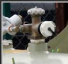
Regulator & filling point
