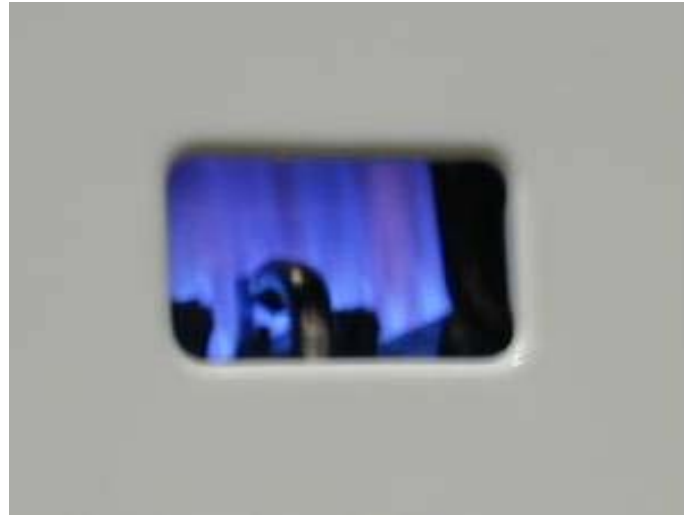
Figure 14: Burner under normal operating conditions
