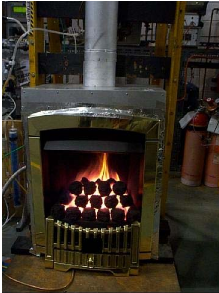
Figure 23: High gas supply pressure fault
