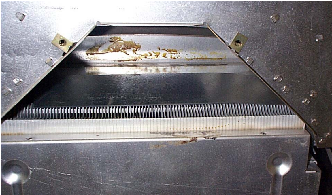
Figure 42: “Close-up” of the blocked heat exchanger
