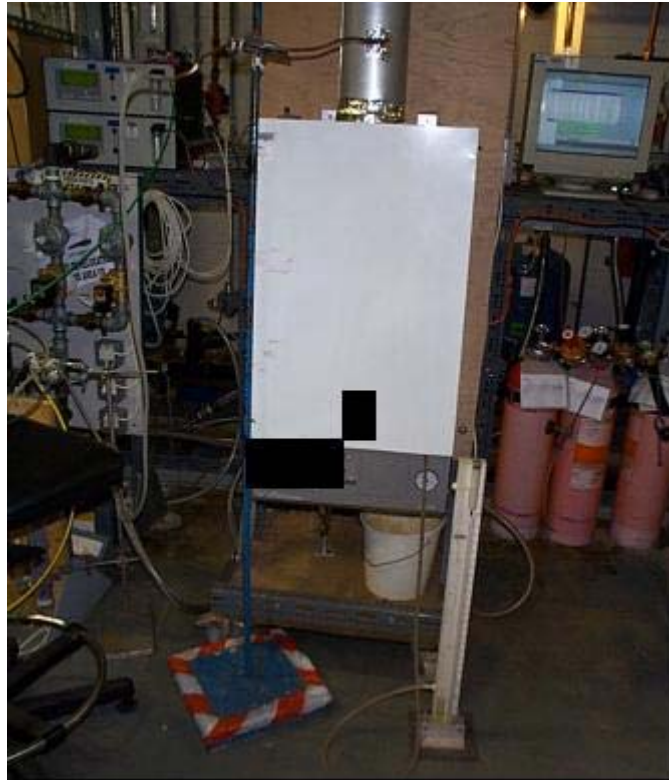
Figure 37: Open flue combi-boiler in the test bay
