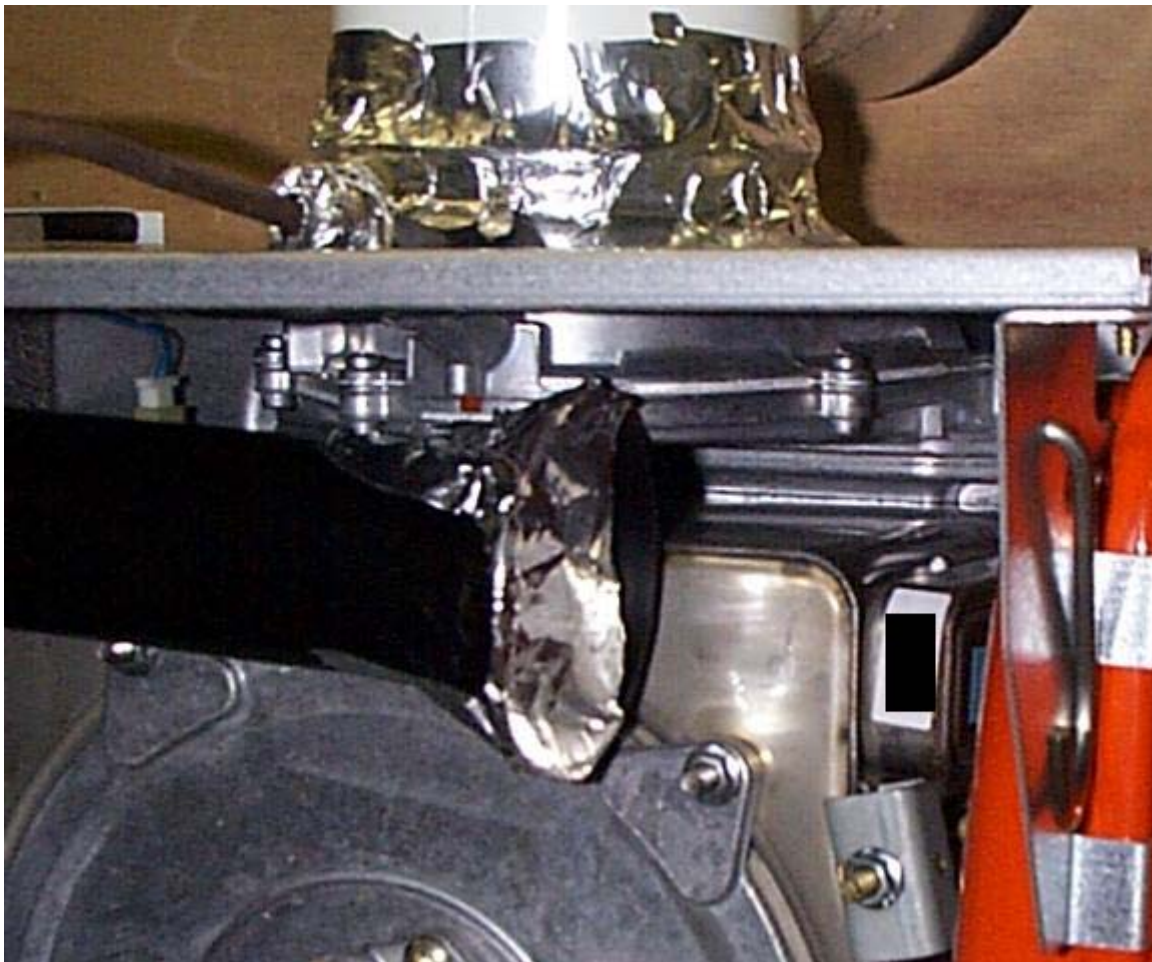
Figure 36: “Close-up” of partially blocked air intake funnel
