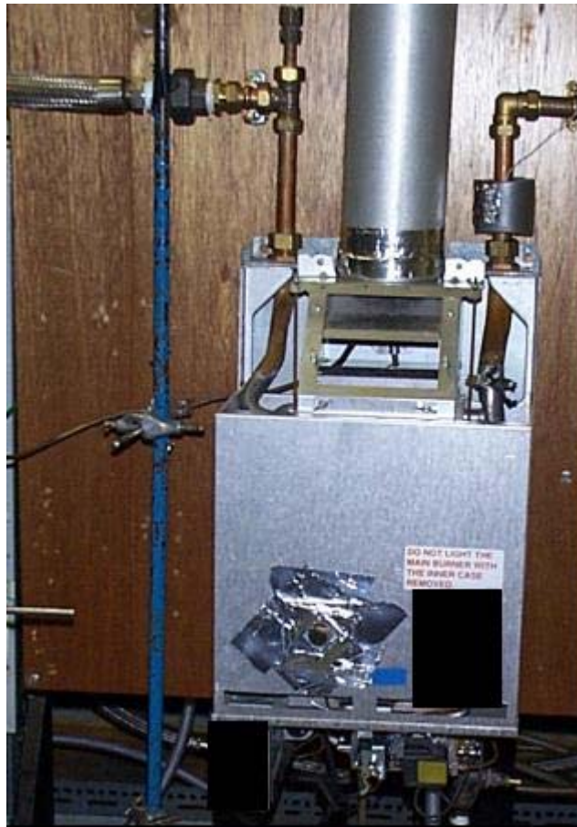
Figure 30: Blocked boiler heat exchanger
