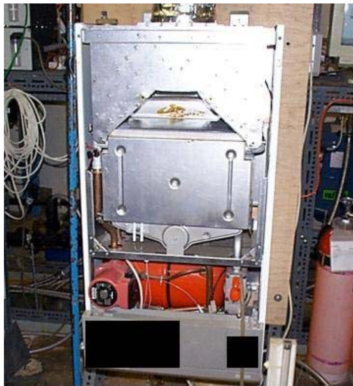
Figure 41: Blocked heat exchanger and internal structure of the combi-boiler
