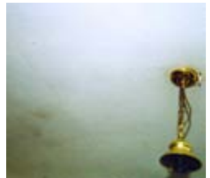
Textured coating with asbestos
