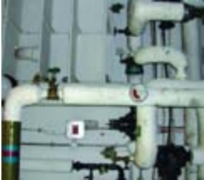
Asbestos insulation on pipes
