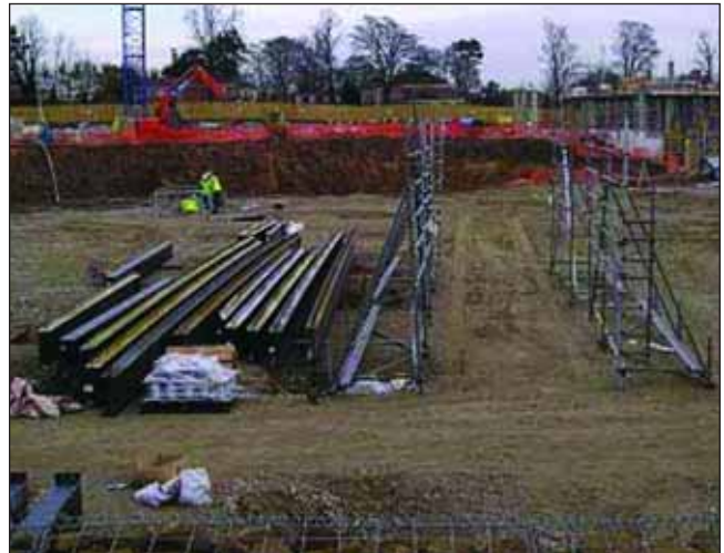
Figure 1 Drive through unloading gantry
