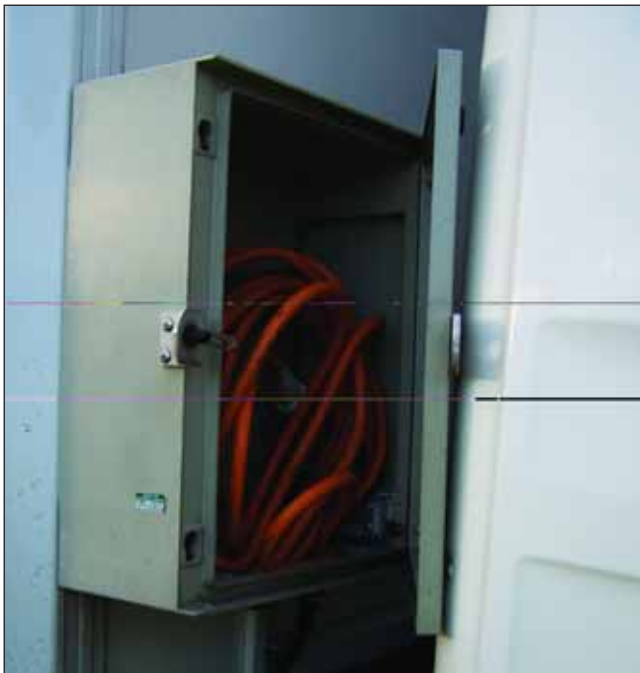
Figure 3 New interlocked trailing leads
