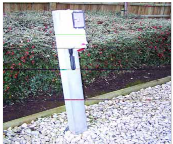
Figure 4 New socket outlets for refrigerated vehicles while parked
