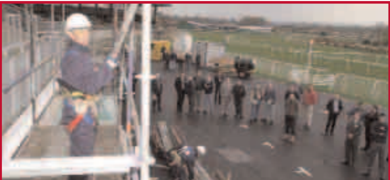
A live demonstration of an easy to erect 'system' scaffold at the SHAD held at Haydock earlier this year
