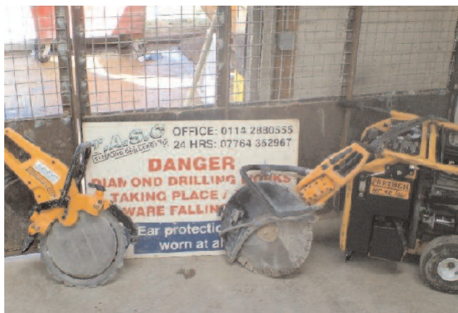
Figure 1 Hydraulic ring saw and power pack. The use of long hoses allowed the cutting equipment to be used 20 m away from the generator, enabling a major noise source to be located away from the operator and others working in the area
