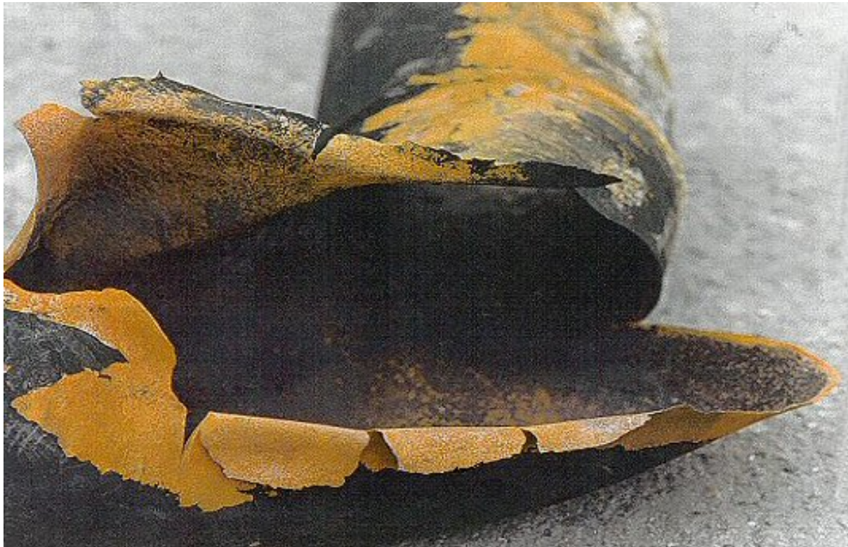
Figure 7 – The failed elbow recovered from the plant
