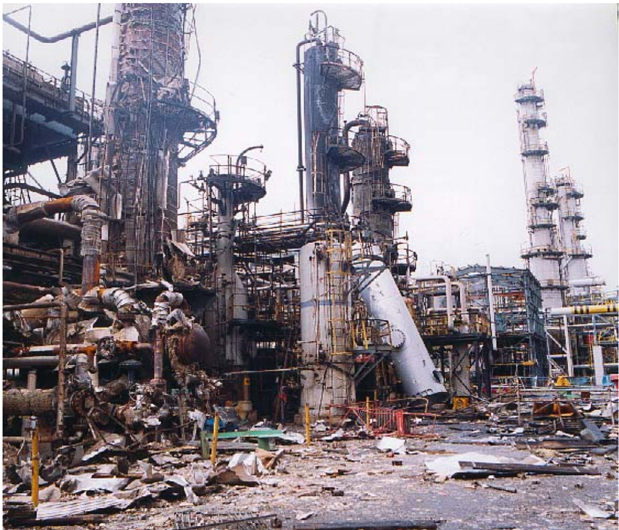
Figure 4 – Damage to adjacent Plant
