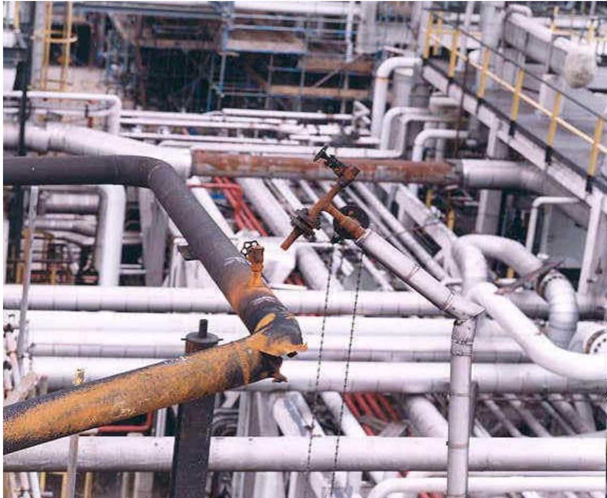
Figure 9 – In-situ failed elbow and injection pipework connection (broken off)
