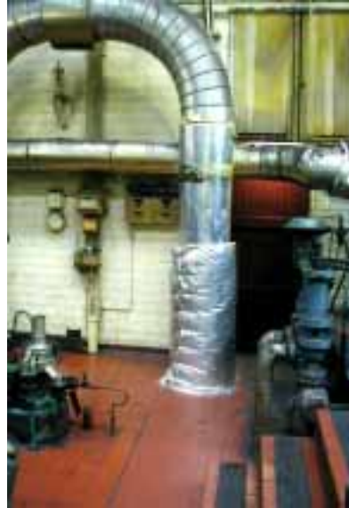
Photo: Aluminium cladding above and to the side of a pedestrian access route where there is a higher likelihood of impact damage.
