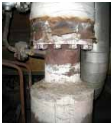
Photo: heat damage to recent asbestos encapsulation
