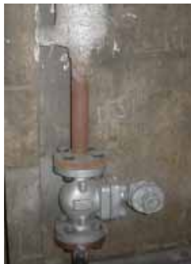
Photo: access is required to maintain the valve, therefore asbestos lagging has been removed from working area.
