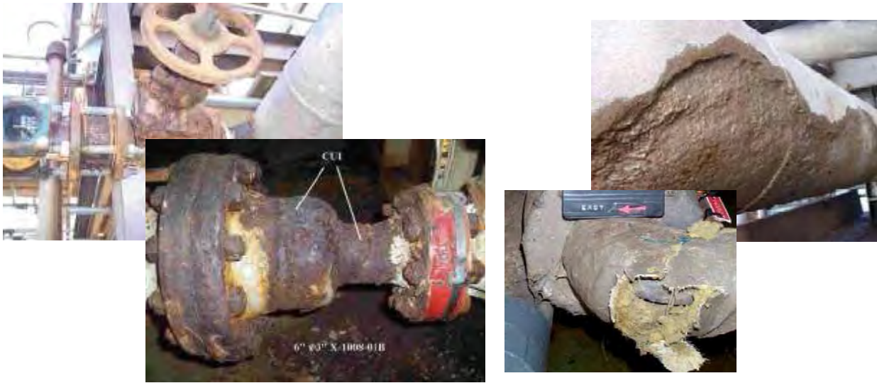
Figure 9: Examples of Corrosion Under Insulation
