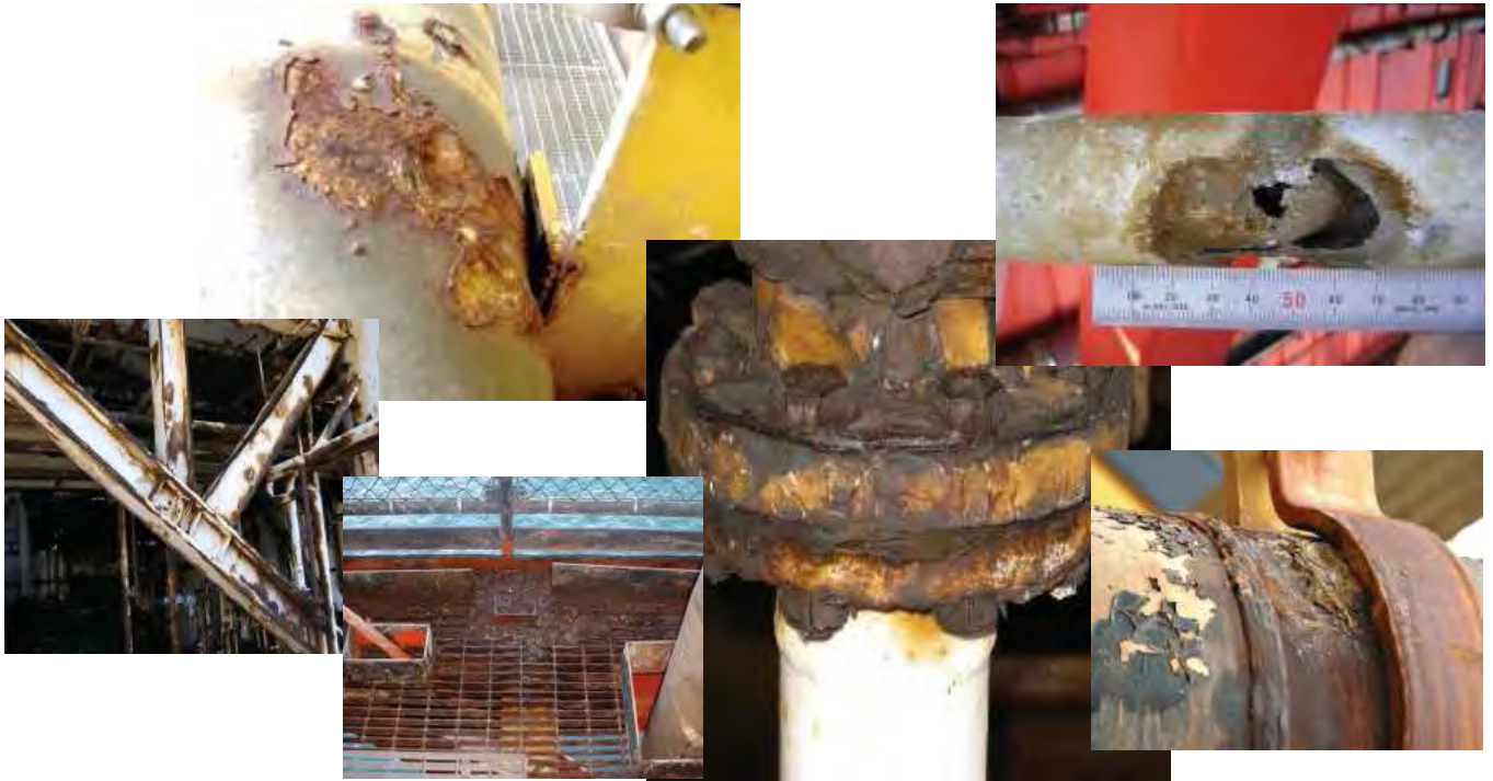
Figure 6: Examples of Atmospheric Corrosion
