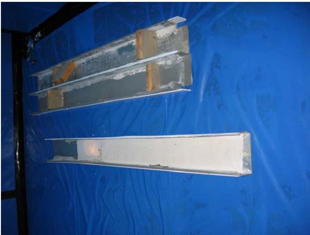
Figure 14: Example of casings removed from columns showing where AIB had been removed or left in place.
