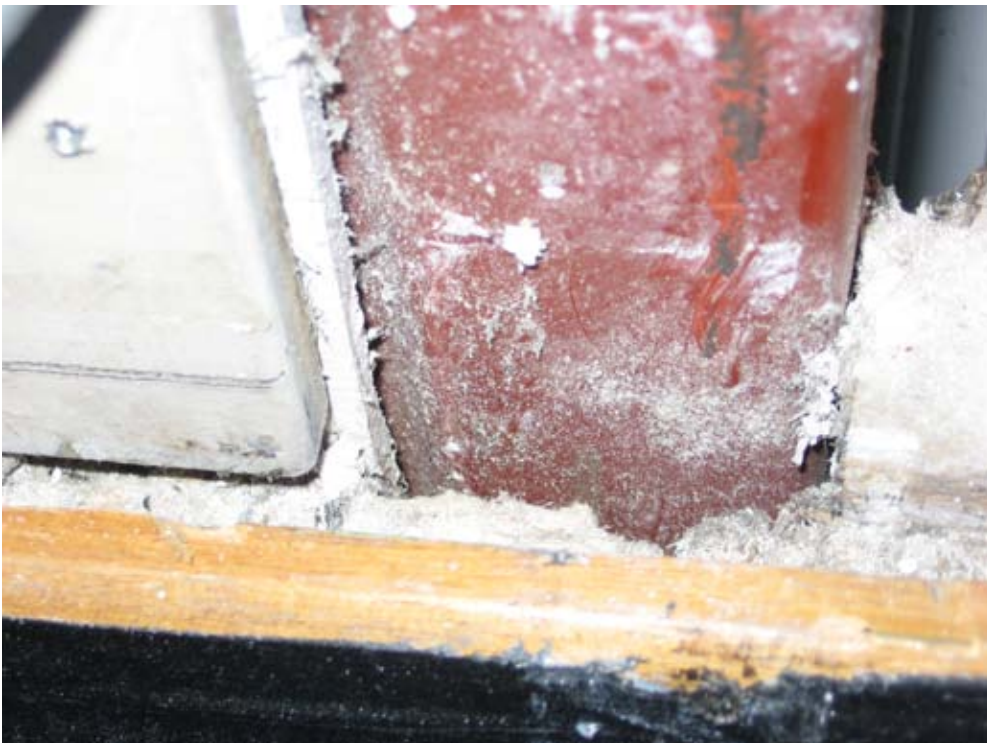
Figure 11: View of base of column from which the casing in figure 10 was removed. A large amount of friable AIB debris can be seen.
