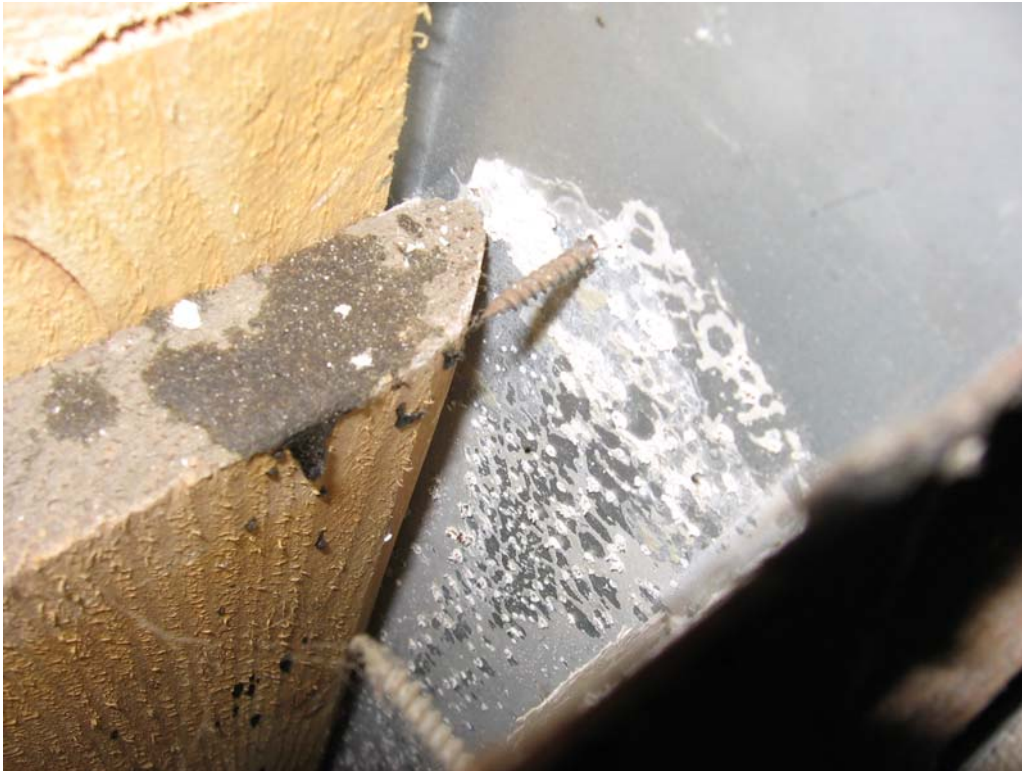
Figure 13: Example of asbestos debris from pieces of AIB that was glued onto the casing but had been torn off at some time. View down the column from above the suspended ceiling.
