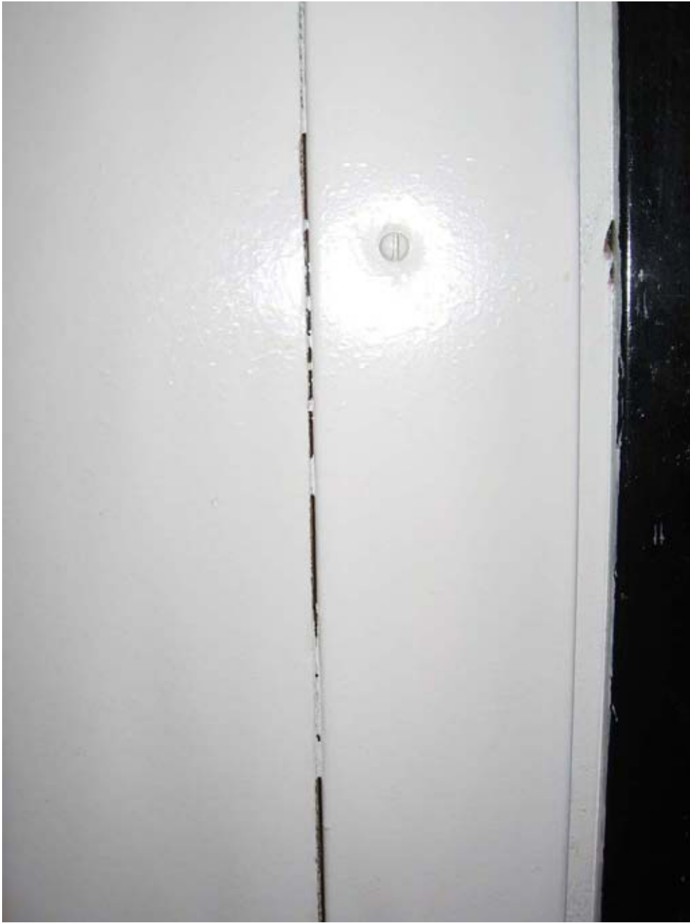
Figure 12: Example of a gap in the casing.
