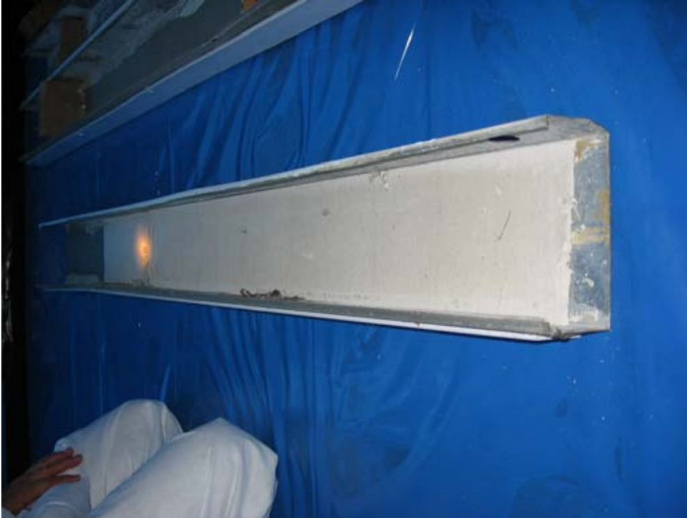
Figure 10: Example of a column casing with AIB attached to one side of the casing. The torch beam shows where the AIB has fractured due to a screw being placed into the casing. A hole is visible in the side of the casing and visible debris shows that friable material was present.
