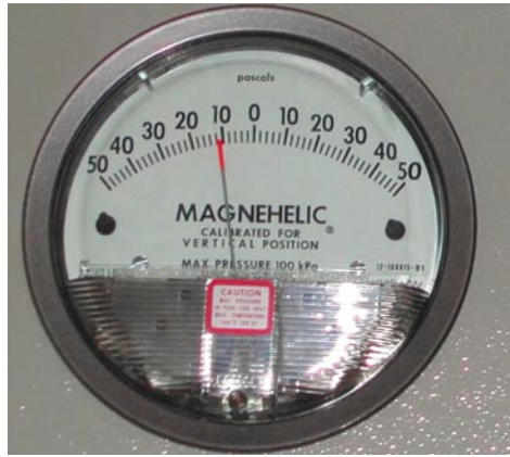
Example of a manometer fitted to a spray booth
