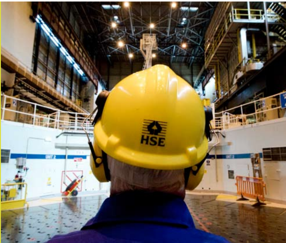
ONR inspector at Heysham 1 Reactor 2 boiler tops, looking towards the refuelling machine connected to Reactor 1
